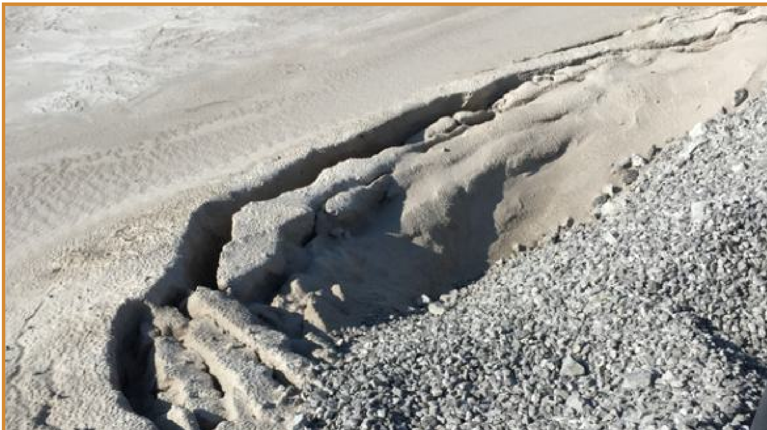
Photo Of On Site Sinkhole
